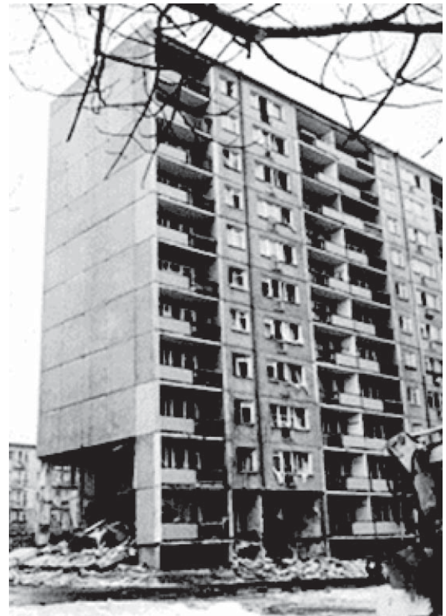
Figure 6 - Effects of a gas explosion in a large-panel building (Łódź, Retkinia housing estate)
