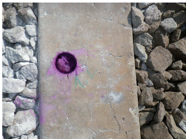
Figure 8 – Cracking on the sleeper produced in 2010
