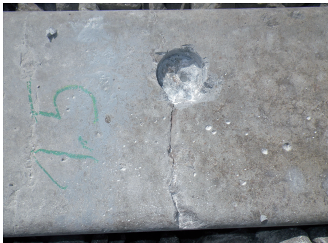
Figure 5 – Cracks within concrete sleeper
