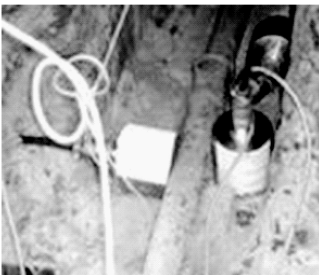
Figure 5 - Vibration sensors № 1, № 2 and № 3 for the registration of foundation oscillations oriented towards X, Z and Y directions
