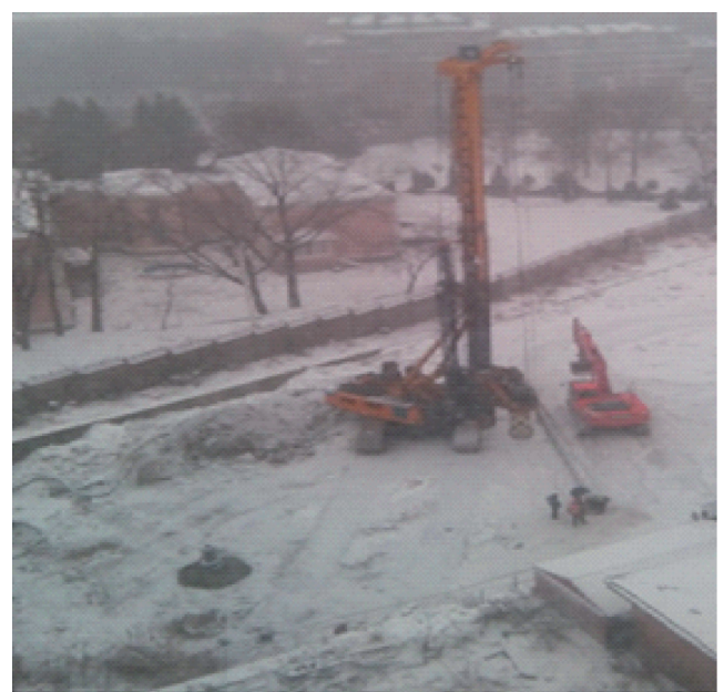
Figure 4 - Construction site located near the building at 14, Pimonenko street (view from the flat on the 9th floor)
